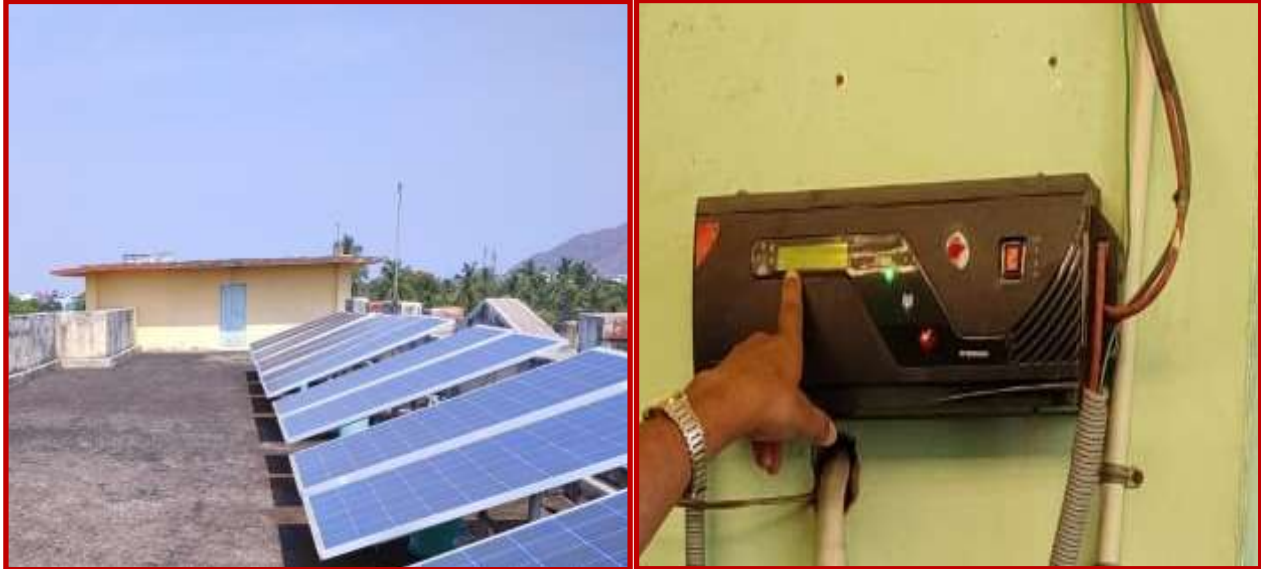
Fig.5: 4-kW Roof Top Solar Plant & Inverter System
