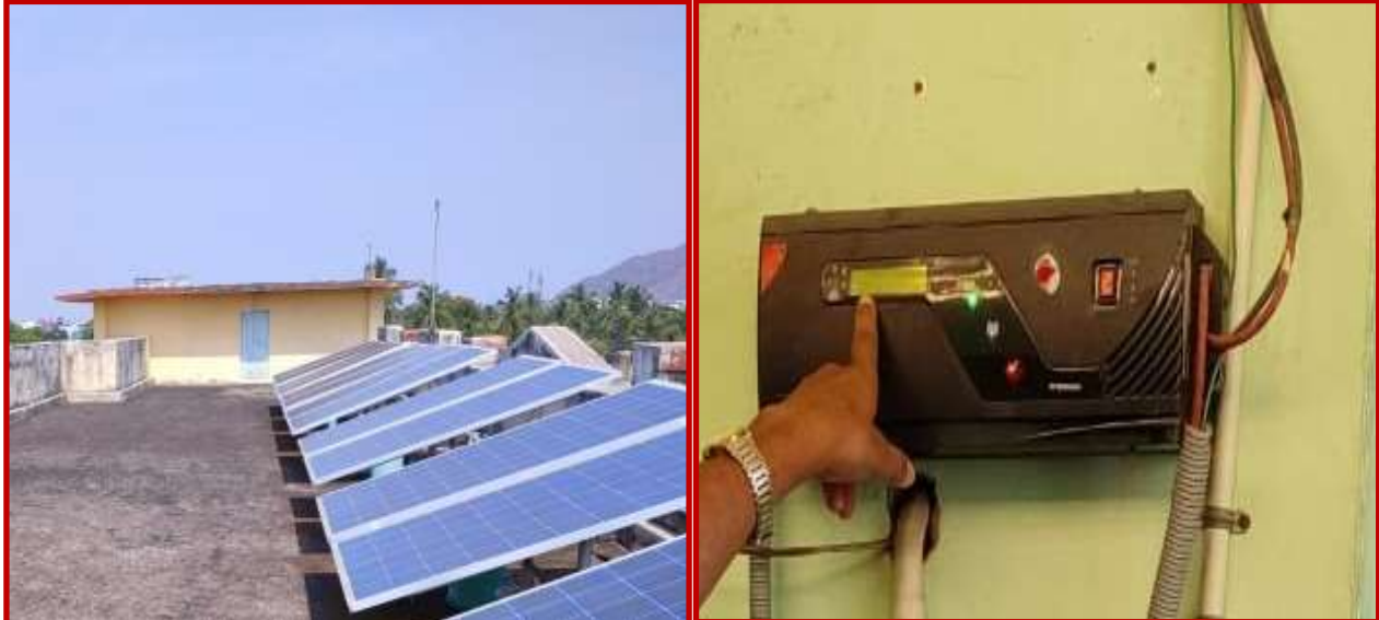
Fig.5: 4-kW Roof Top Solar Plant & Inverter System
